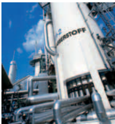
Linde-Steamreformer in Burghausen
